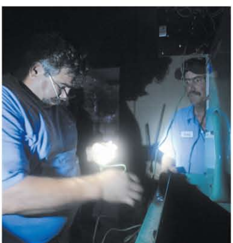
Freeport Mayor Larry McDonald, left, works on a generator as city employee Scott Rogers holds a flashlight for him Friday night at the Freeport Police Department. The power went out at the police department about 6 p.m. Friday and the generator that normally would power the building in an outage also was not functioning.
